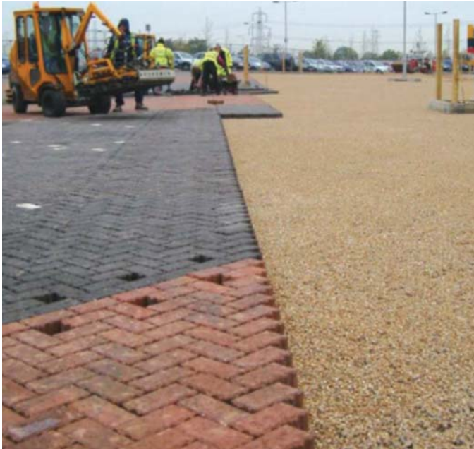
Machine laying of concrete paving units offers a particularly efficient solution for permeable as well as conventional block paving.
