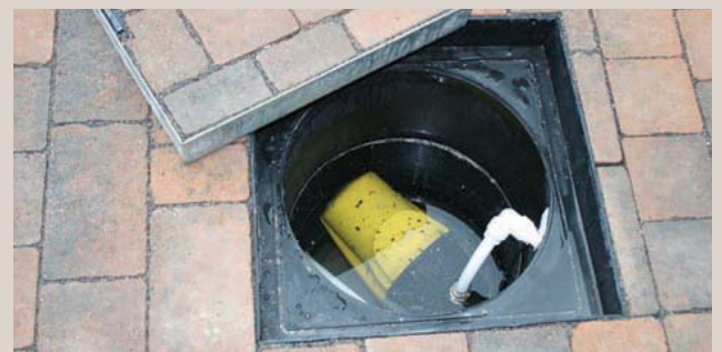
Around this home, rainwater runoff collected from all impermeable surfaces including roofs and paths, together with the 60m 2 permeable drive itself, passes into the tanked permeable pavement which contains a concealed sump. Here, a small pump is used to draw off the harvested water, in this case for outside uses, via a tap and hosepipe.
